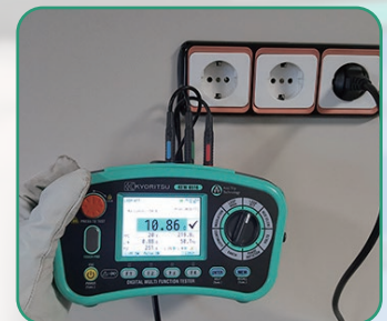
Loop test from a wall socket
